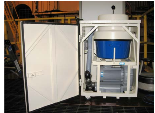
Cooling system – vacuum
